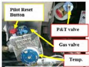
Water Heater pilot ignition
