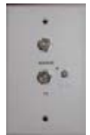
Antenna Power Supply
